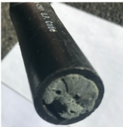
Melted and re-hardened plastic inside pipe w/ different color
