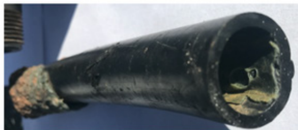
Whole view of pipe A with A melted plastic inside (A1) and melted plastic on outside (A2)
